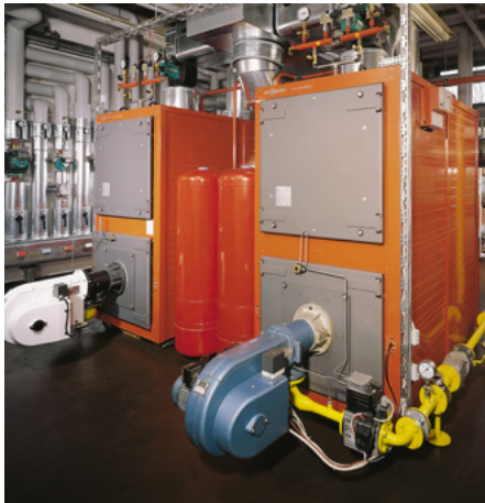
Gas inlet pressure monitoring on high-performance boilers
