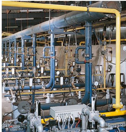
Gas train in a brickworks
